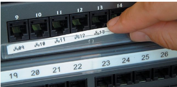
Punch block & patch panel labels
